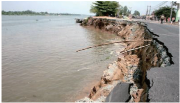
Fig.10 River bank erosion in the Mekong Delta
